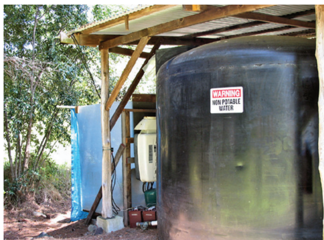
Figure 11.7 —A backup water storage tank containing sufficient water to meet the nursery's needs for at least 1 week is a prudent investment. Photo by Thomas D. Landis.
