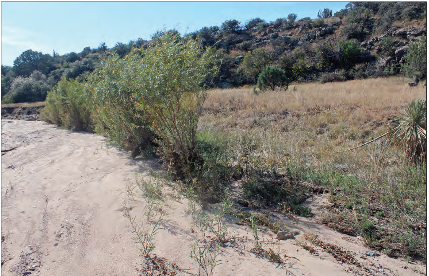
Figure 3. Coyote willows planted in 2012 armor a bank at the top of Walking X Canyon. Four years later, erosion has been mitigated, grass has been reestablished on the bank, and the willows have put out numerous suckers. (Photo by Erin Evans, 2016)
