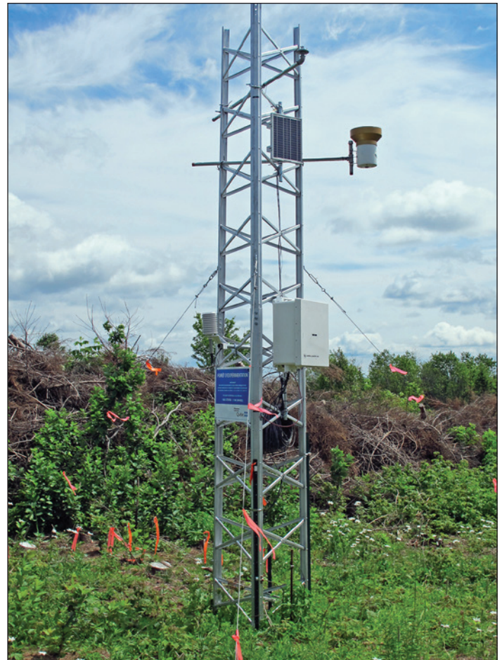
Figure 2. A permanent meteorological station was installed April 2013 at the Watford plantation site (Photo by Mohammed S. Lamhamedi, July 2013)
