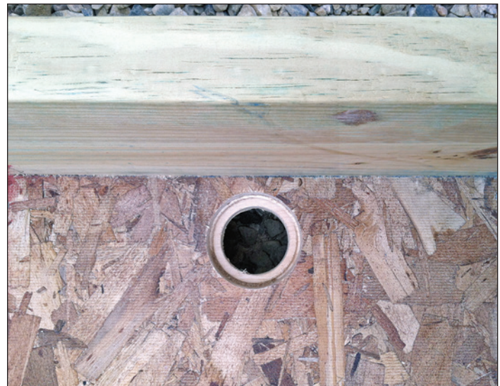
Figure 6. Drain assembly for subirrigation tank using a 1-in heavy duty polypropylene tank fitting with a 2.25-in hole size. (Photo by Tammy Parsons, 2015)
