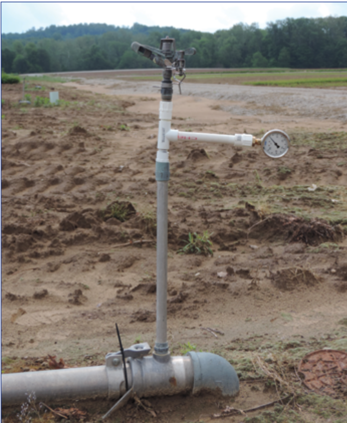
Figure 4. Measuring water pressure with a pressure gauge installed on a riser. (Photo by Ronald Overton 2014)
