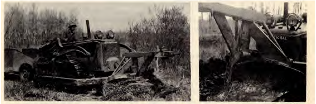
Minnesota pusher plow ahead of a TD-9 tractor. Planting machine is pulled behind tractor at the same time.
