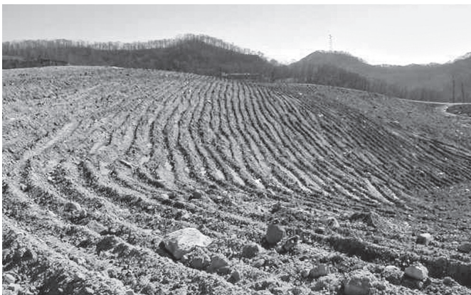
Figure 2. A single shank ripper pulled by a D11 was used on this gently sloping area to a depth of \approx 2 m on the University of Kentucky's Bent Mountain Reforestation Research Complex in Pike County, Kentucky. Surface water retained in the rips reduces runoff, erosion, and sedimentation.
