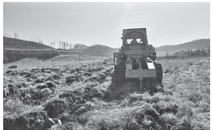
Figure 1. Single shank ripping with a D9 dozer on an abandoned surface mine site near White Oak, Tennessee.
