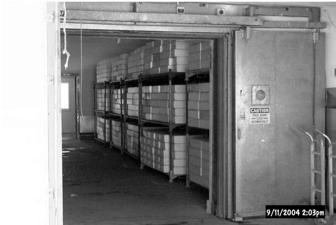
Figure 9 —A storage cooler was converted into a sterilization room. Steam pumped into the room provides high-humidity heat.
