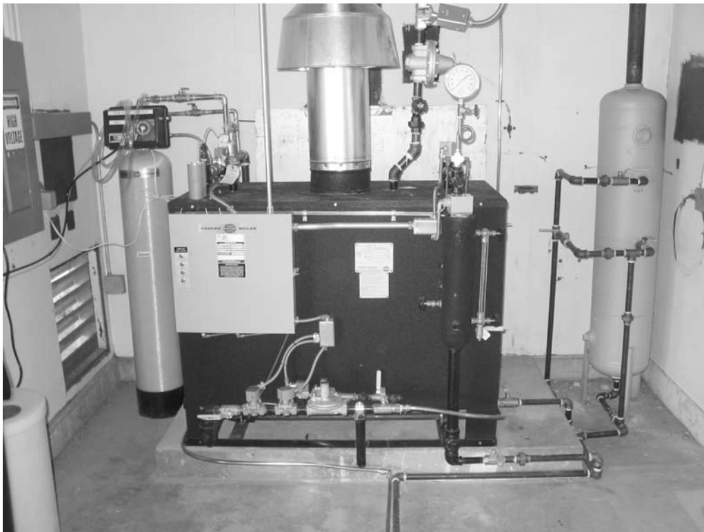
Figure 10—A 9.5 hp steam boiler was used to heat the sterilization room.
