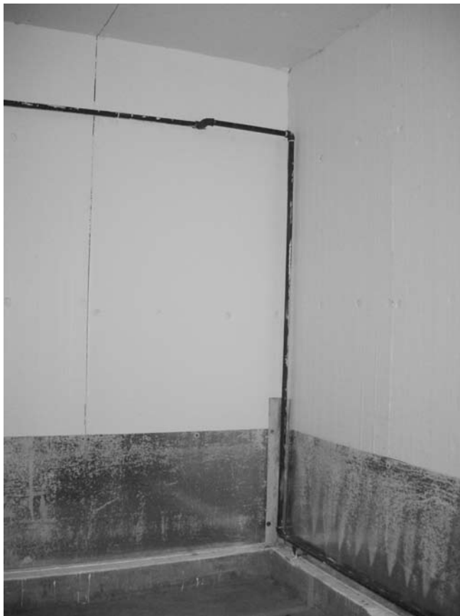
Figure 11 —Black pipe distributes steam in the sterilization room. The pipe runs along the bottom of the side walls. Steam leaves the pipe through holes (0.06 in [0.15 cm] in diameter) drilled into the pipe.
