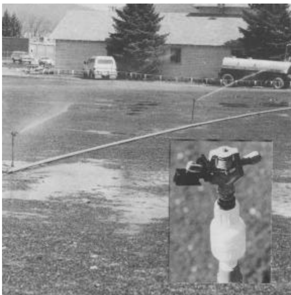
Figure 10. Impulse sprinkler systems (sprinkler head shown in inset) have adjustable water trajectories and rotation patterns.
