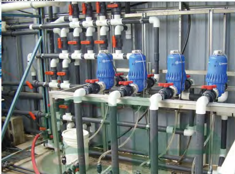
Zwart Systems controls multiple 40 GPM Dosatrons for different water flow rates.
