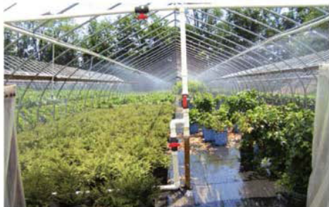
The pumps are most effective and economical when there is a considerable difference in demand between large irrigation zones.
