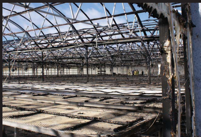
Combustible components and materials stored within the greenhouse act as fuel. It's important to identify what will be "fuel" if a greenhouse fire were to start.
