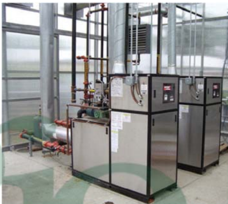
Boilers can provide modulated water temperature for root zone heat during spring and fall greenhouse operation.
