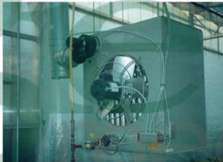
Unit heaters along with horizontal air flow circulation provide uniform heat. This system is good for greenhouses closed during the winter as the system does not have to be drained.
