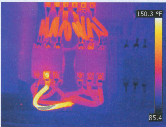
A closer look at these starter connections also reveal a significant hot spot with the bright yellow connector.
