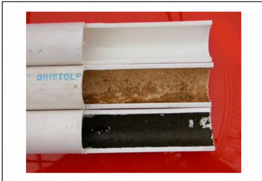
Figure 7. Longitudinally cut PVC mains; top section is new, middle section carries clear water, bottom section carries fertilizer. Note discolored biofilm layer in clear section and algae dominated layer in bottom section.
