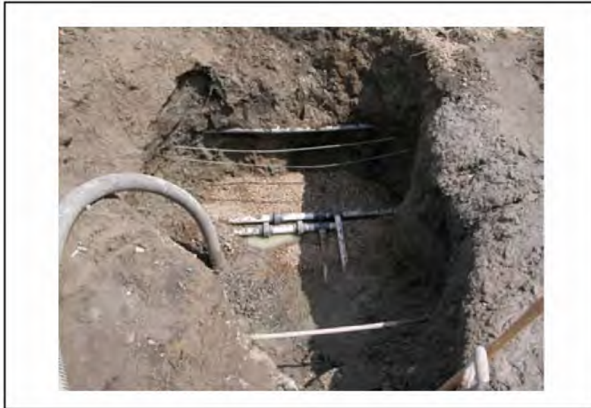
Figure 6. Underground clear water and fertilizer mains, which were cut to show algae and biofilm growth in the absence of sunlight.
