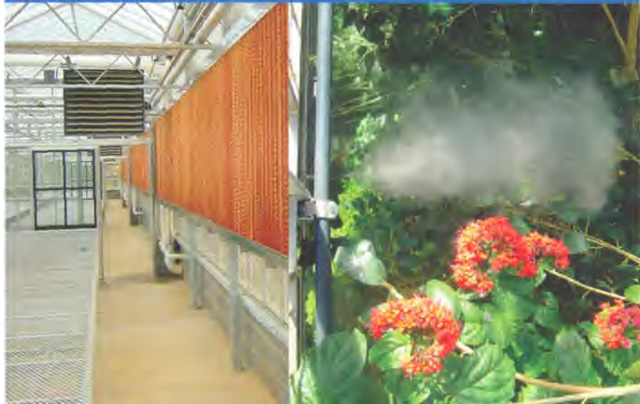
Two evaporative cooling systems are commonly used in greenhouses: pad-and-fan (left) and fog (right).
