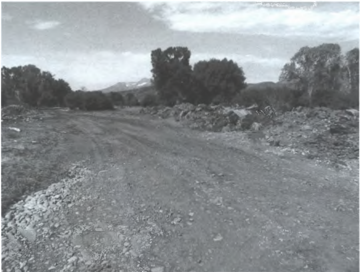
Figure 2—P R R P haul route. Note that the top foot of soil, which contains plant roots and seeds, has been stockpiled to the right of the road. This minimizes handling of the topsoil. Decommissioning of the route would follow the sequence of removing any road fill, grading to establish proper contour, ripping (if necessary), and replacement of topsoil.
