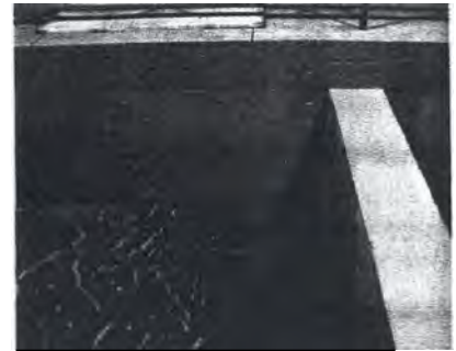
Concrete water-holding tanks can be chemically sealed with epoxy to prevent microbial organisms from taking up residence in the concrete's pores.
