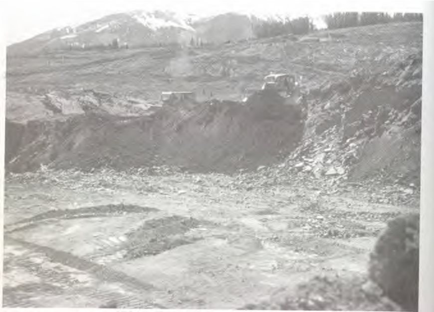
Fig. 21-5. Selective handling of soil materials is not practical in the alpine and subalpine. Soils are salvaged in one lift.
