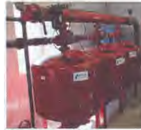
Use of sand filters is increasing, particularly in operations drawing water from ponds.
